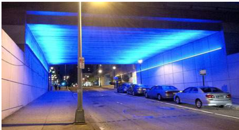
Decorative LED lighting provides aesthetics & pedestrian comfort to highway overpass
